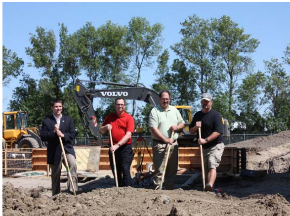
Pictured (left to right) Jasper Schneider, State Director of USDA Rural Development, Don Frye, mayor of Carrington, Randy Pope, Interstate Engineering and Brian Herrington, Carrington water plant supervisor, move a ceremonial first shovel of dirt on the new water treatment project at Carrington.
