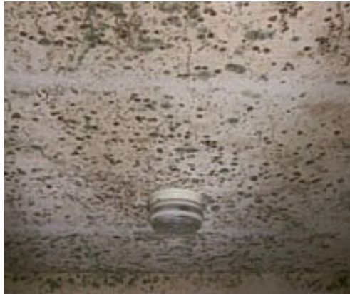
Mold on a ceiling around a smoke detector
