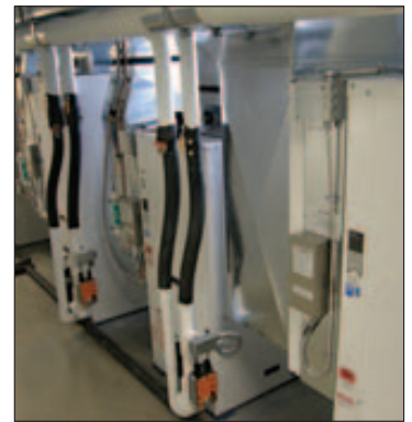
TEMPERATURE CONTROLS: With a geothermal system the temperature inside the building is controlled by nine heating and cooling zones.
