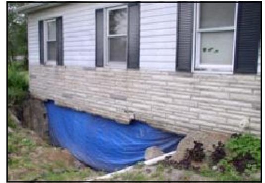
Karlyon Jones of Coulterville, Illinois turned to USDA Rural Development for help when 24 feet of her basement collapsed a few months ago.
