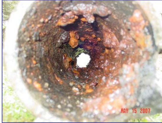
This picture illustrating an aging pipeline was provided by Brian Tarbuck, General Manager of Augusta Water and Sewer Systems. A more detailed description is provided on page 7.
