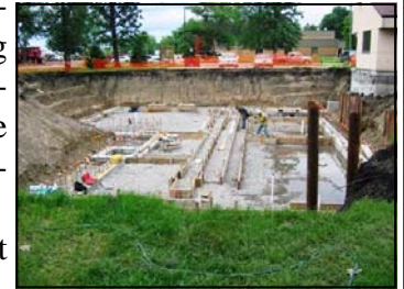
Construction is underway on the addition to the Northwestern Mental Health Center.
