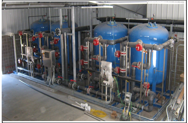
AdEdge Arsenic Removal Equipment.
