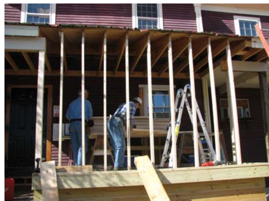
Contractor, John Thompson, and his long-time employee, Bob Woodward, are building the deck and exterior walls for OCC's walk-in refrigerator/freezer.
