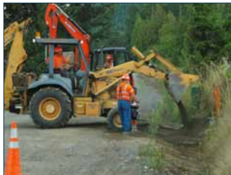
Toledo Telephone Company's "Last Mile" fiber optics expansion project in Lewis County. Photos by Phil Eggman.
